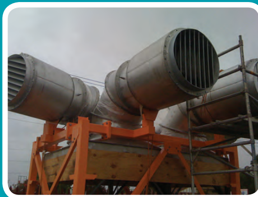
Offshore Condenser Fans
